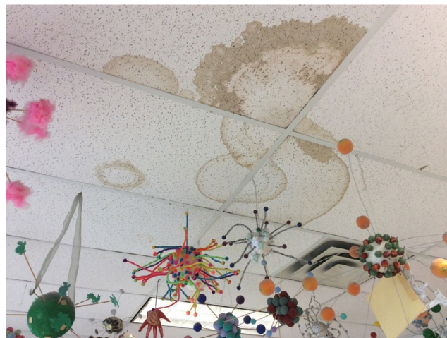
FIGURE 1 An example of visual evidence for mold growth due to water damage from water pipe leakage on a classroom ceiling. This was commonly observed at multiple schools
